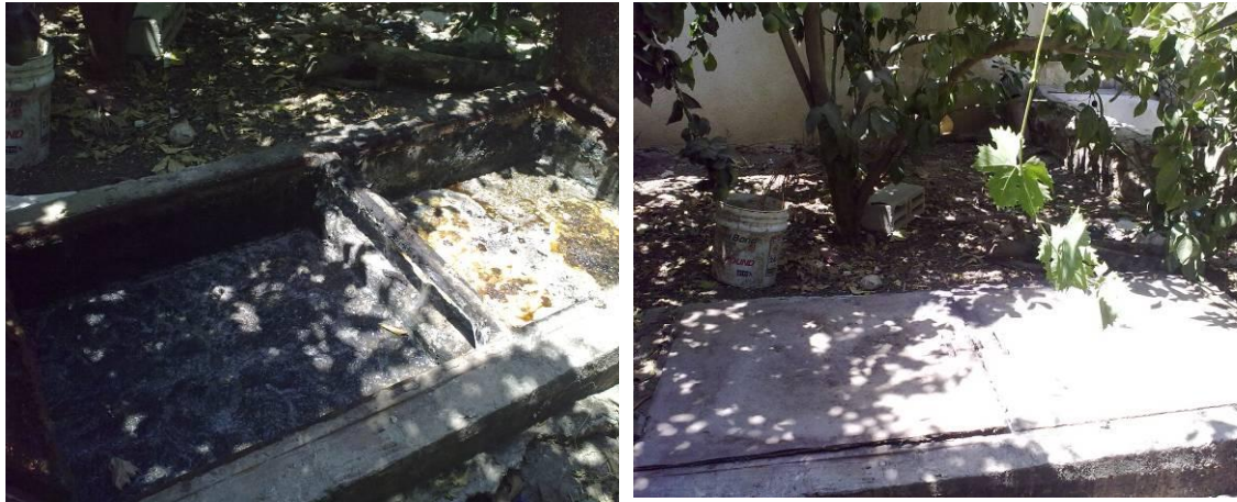
Photo B.11 Household onsite Upflow Gravel Filter wastewater treatment plant in Sanur Village in Jenin Governorate
