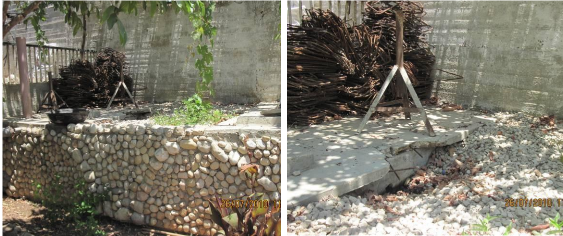
Photo B.14 Household onsite Upflow Gravel Filter wastewater treatment plant in Qibya Village in Ramallah Governorate. Right photo shows penetration in the septic tank which leads to allow entrance of air to be aerobic tank instead of anaerobic status.
