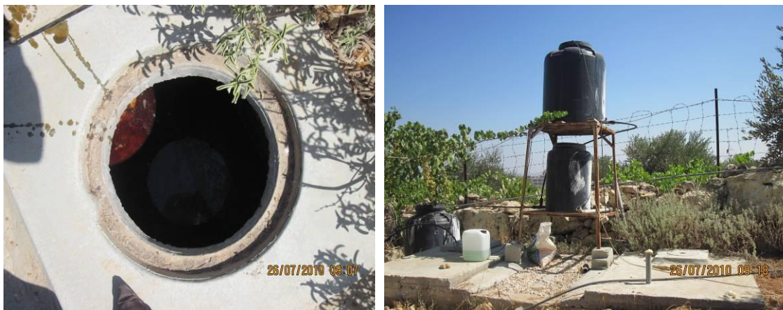
Photo B.13 Household onsite Upflow Gravel Filter wastewater treatment plant in Beit Anan Village in Jerusalem Governorate. Left photo shows accumulation of oils in the
