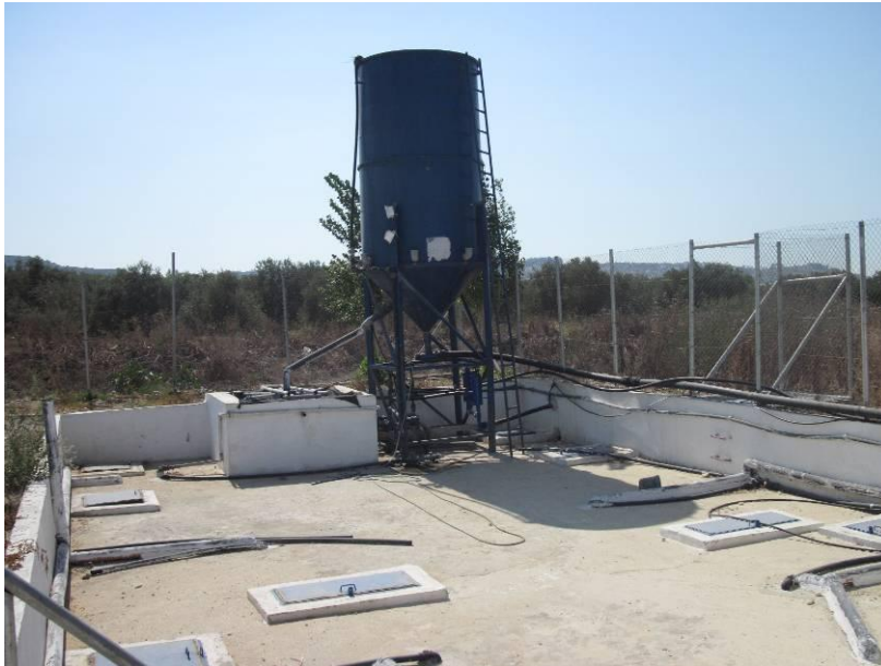
Photo B.3 Collective onsite wastewater treatment plant consists of Septic Tank - Anaerobic Upflow Gravel Filter - Aerobic Trickling Filter followed by Polishing Sand Filter located in Attil Village in Tulkarem Governorate
