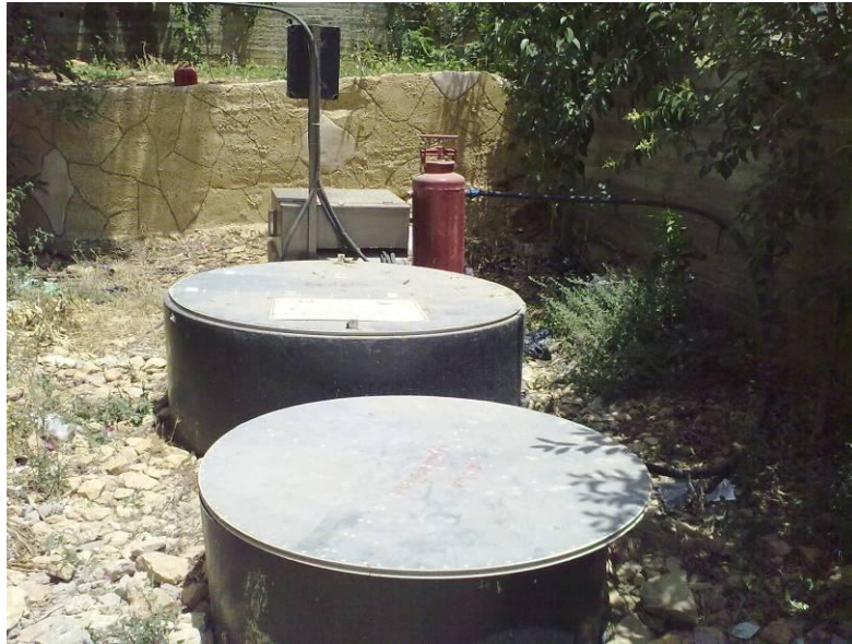
Photo B.9 Household onsite Activated Sludge wastewater treatment plant in Beit Omer Village in Hebron Governorate
