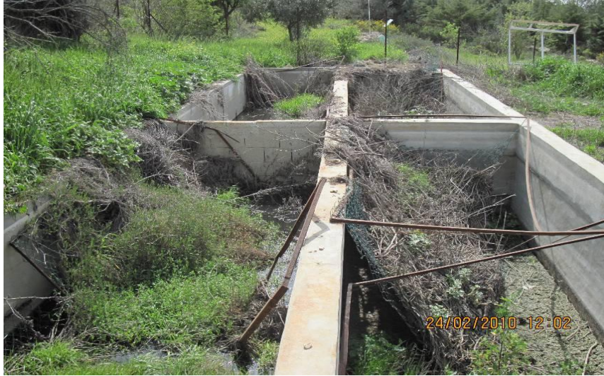
Photo B.1 Community onsite of waste stabilization bond located in Talita Kumi Shchool in Beit Jala.
