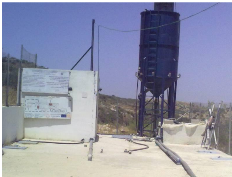
Photo B.4 Collective onsite wastewater treatment plant consists of Septic Tank - Anaerobic Upflow Gravel Filter - Aerobic Trickling Filter followed by Polishing Sand Filter located in Sir Village in Qalqilya Governorate
