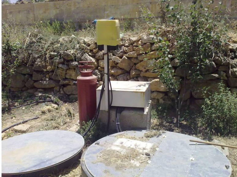
Photo B.7 Household onsite Activated Sludge wastewater treatment plant in Battir Village in Bethlehem
