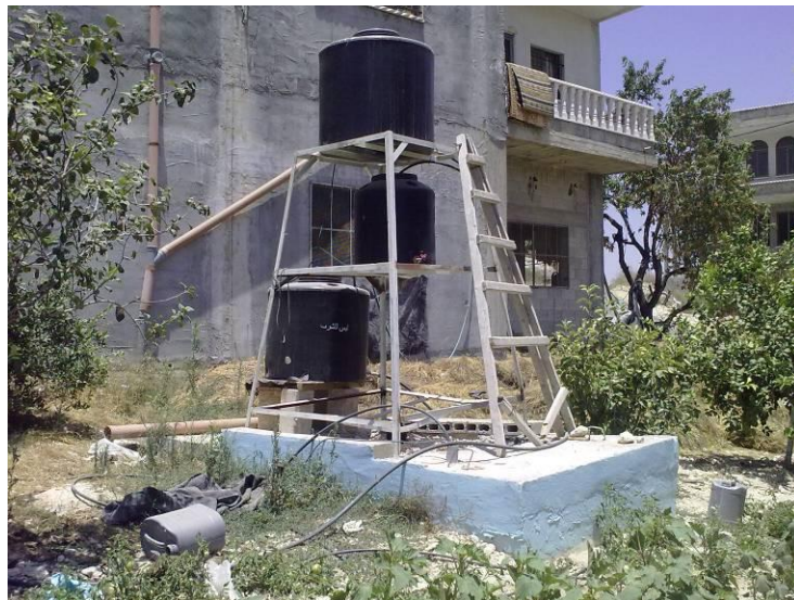
Photo B.12 Household onsite Upflow Gravel Filter wastewater treatment plant in Beit Leed Village in Tulkarm Governorate
