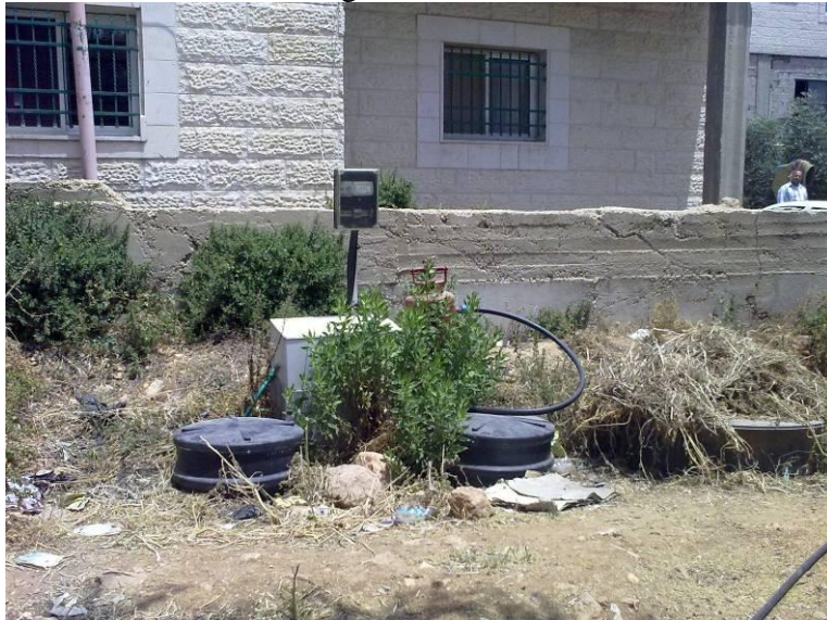
Photo B.8 Household onsite Activated Sludge wastewater treatment plant in Nahalin Village in Bethlehem
