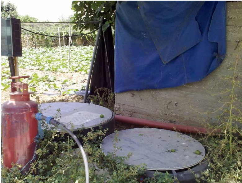
Photo B.10 Household onsite Activated Sludge wastewater treatment plant in Halhul Village in Hebron Governorate
